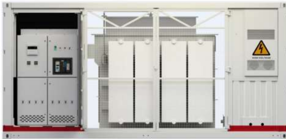
Figure 7 the Front View of STS-6000K Transformer station
