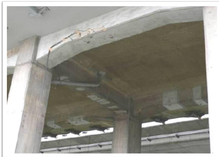
Figura 2. 8. Vigas de viaducto Suda K., R. K. (2005). Anti-Carbonization Process Utilizing Direct Sprayed ECC Applying to Railway Viaduct Involving Flexural Fatigue Cracks. Concrete Journal , 43 (5), págs. 162-167.
